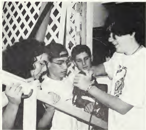
↑“Watch your hands!” Senior Jamie Ford and juniors Steve Brown, Max Kolb and Jonathan Bursell make repairs to a railing.
